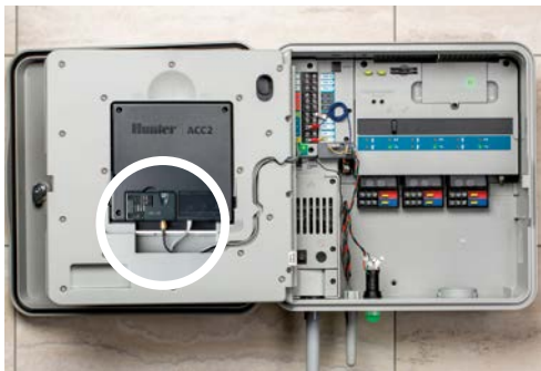
ACC2 Controller with A2C-LTE Module installed
